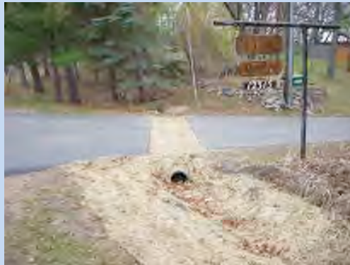
A strategically placed culvert directs water under the asphalt driveway into a natural depression. Prior to the project, all runoff (from County Road 11 and upstream properties) flowed down the impervious driveway and into Big Carnelian Lake.
