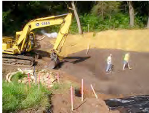
This specially-landscaped area will capture and filter stormwater flowing off of Highway 95.
