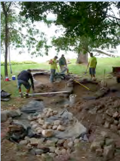
A series of raingardens were installed to address an erosion issue on Big Carnelian Lake.
